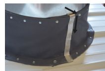
Temporarily fasten strips at bottom. Bend strip down from top over joint
