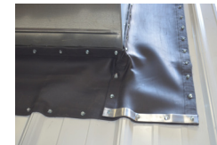
Apply construction grade sealant, appropriate for material surface, along edge to form ramp to slow water flow
